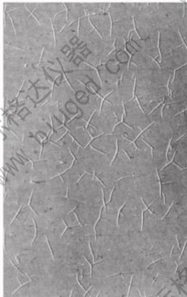
Figure 5 — Crow's foot cracking
